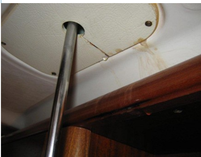
Fig 1(a) – Water ingress into the main saloon
